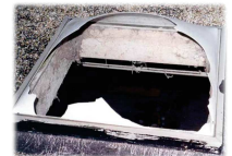
NIOSH FACE Skylight Fatality
