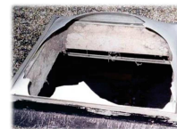
NIOSH FACE Skylight Fatality
